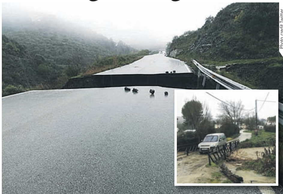
SWAMPED: Rural road damage and flooded streams.
